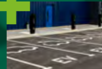
Fast car charging (EV)
